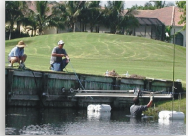
With DSMS technology ... Installations are performed from the waterside of the retaining wall. There's no costly damage to your course and installation time is MUCH quicker.
